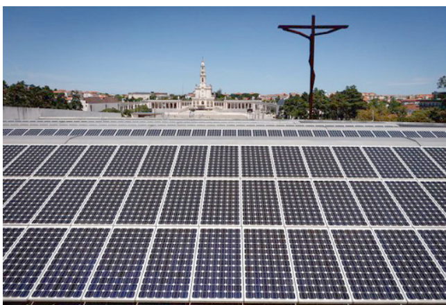
Figure 12: Solar panels installed on top of the Basilica of the Holy Trinity, overlooking the Basilica of Our Lady of the Rosary of Fatima used as an illustration in a report of Laudato Si' research in Portugal .
